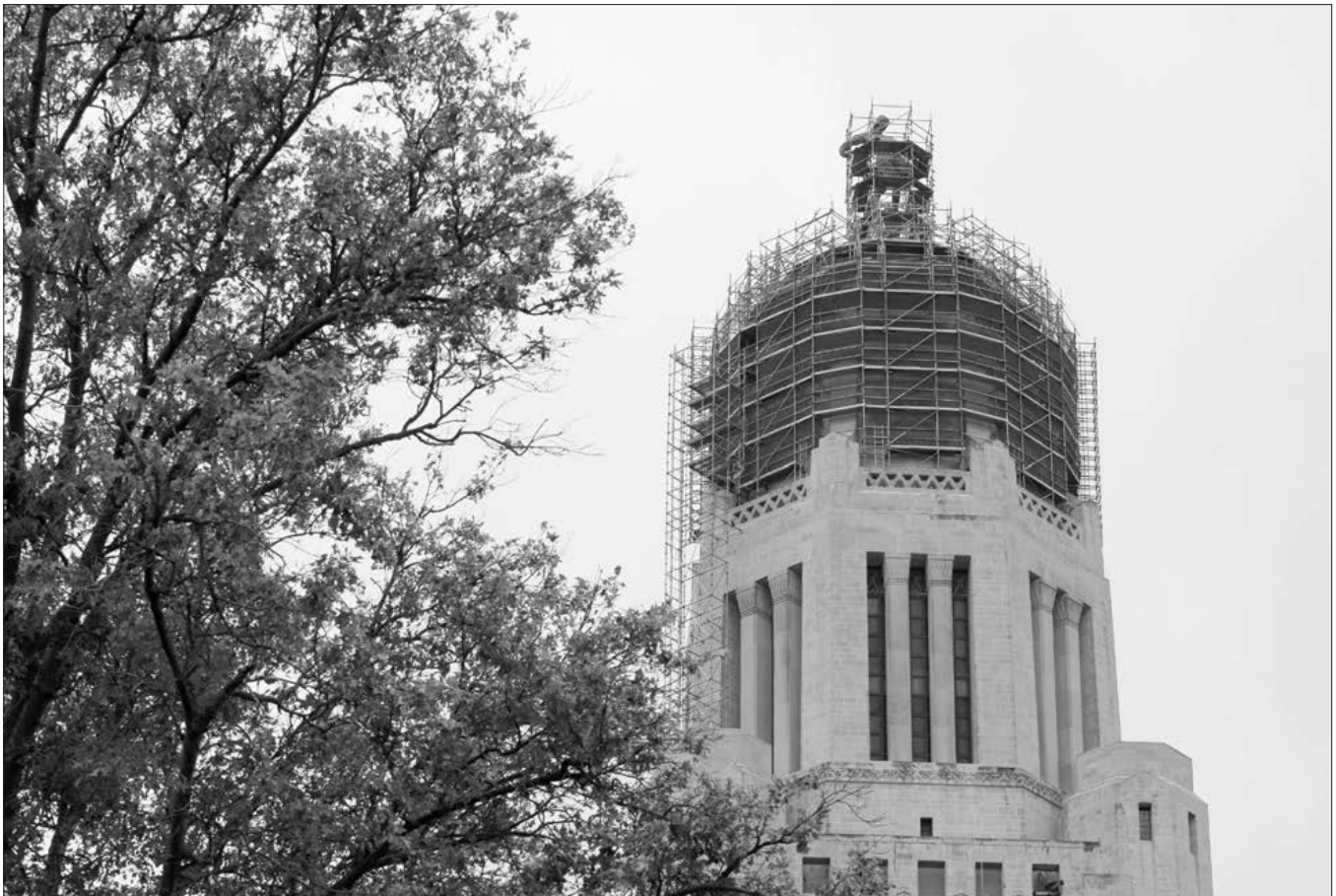
The top of the Nebraska State Capitol is wreathed in scaffolding as restoration work continues on the gold-tiled dome.
