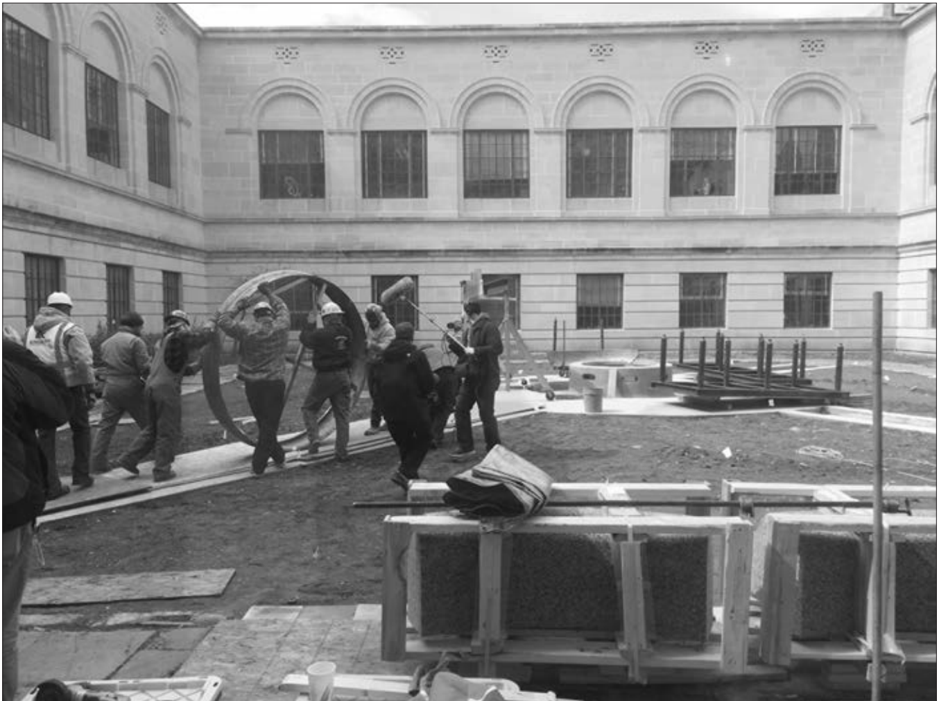
A cast bronze skirt for a Capitol fountain is rolled into the center of the southwest courtyard March 15. Fountains are being installed in each of the four courtyards this spring, completing the final component of architect Bertram Goodhue's original design for the Nebraska Capitol.
